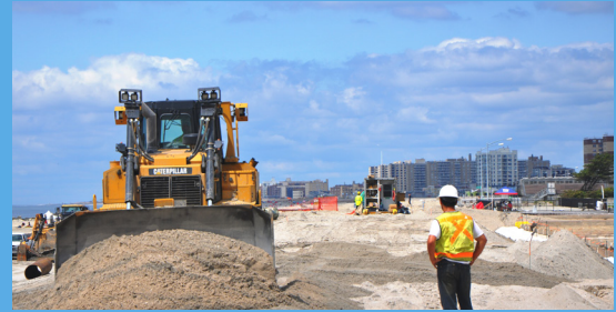
A bulldozer levels sand on Rockaway Beach, Queens, New York, after Superstorm Sandy. Source: John D'Ambrosio, USACE NY
