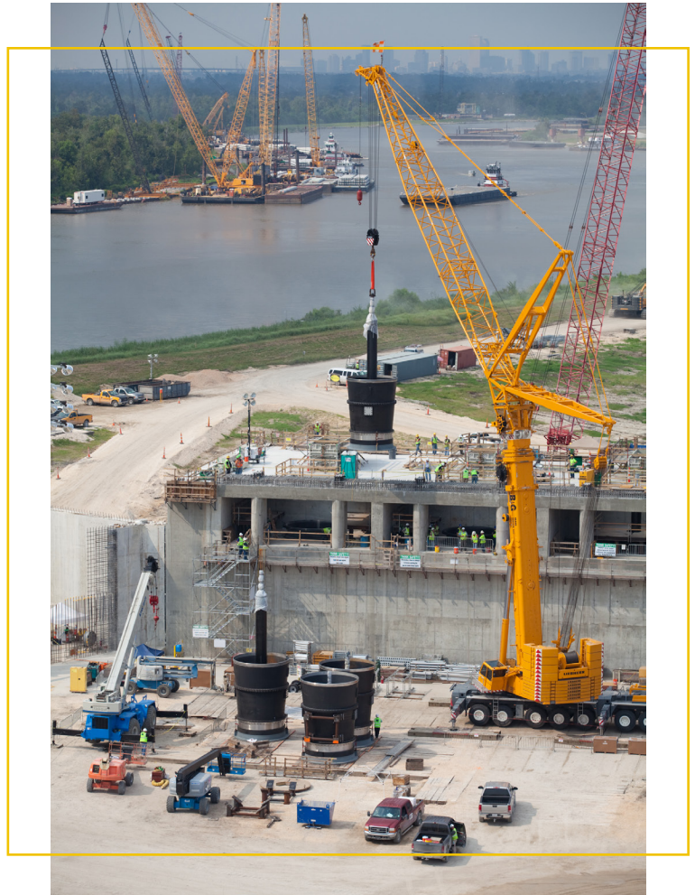
The company Pentair custom-designed 11 pumps for the Gulf Intracoastal Waterway West Closure Complex (GIWW) to protect the city from storm surge.
