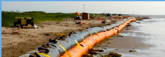
The Louisiana National Guard constructs a diversion system to protect wetlands. Source: Tarell J Bilbo, U.S. Army
