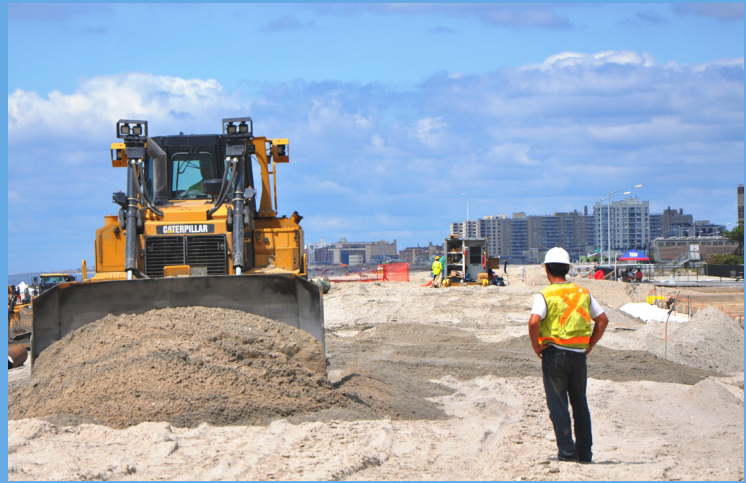
A bulldozer levels sand in Rockaway Beach in Queens, New York, after Superstorm Sandy. Source: John D'Ambrosio, U.S.ACE NY
